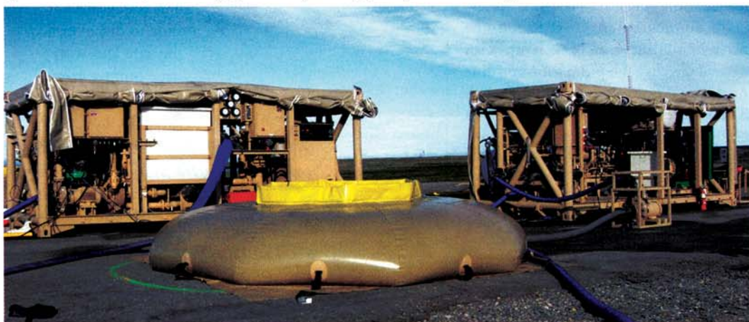
An ultra-filtration (UF) backflush and reverse osmosis (RO) feed tank is positioned in front of an ultra-filtration module (on left) and a reverse osmosis module (on right, with a pump beside it).
